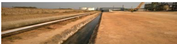
Figure 1: Main drain collector of factory water(Figure 1 : Storm Water Dam)
